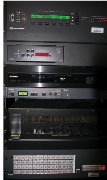
Equipment rack in the Liberal Arts Building's Master Control Room, which interconnects the building's A, B and C sections.
